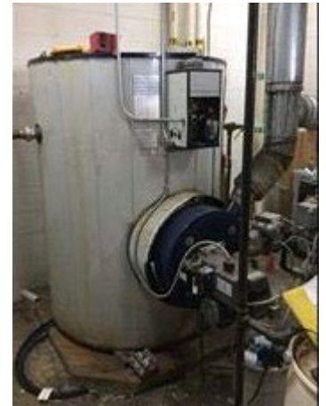
Boiler at Blackfeet Dormitory in Montana
